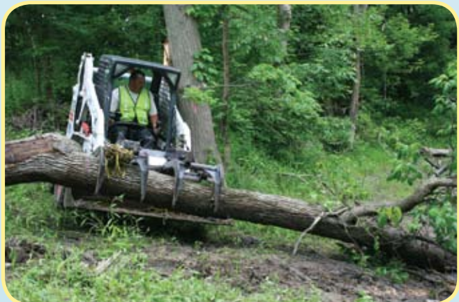
Figure 12 - Be careful not to damage live trees or vegetation with heavy equipment
