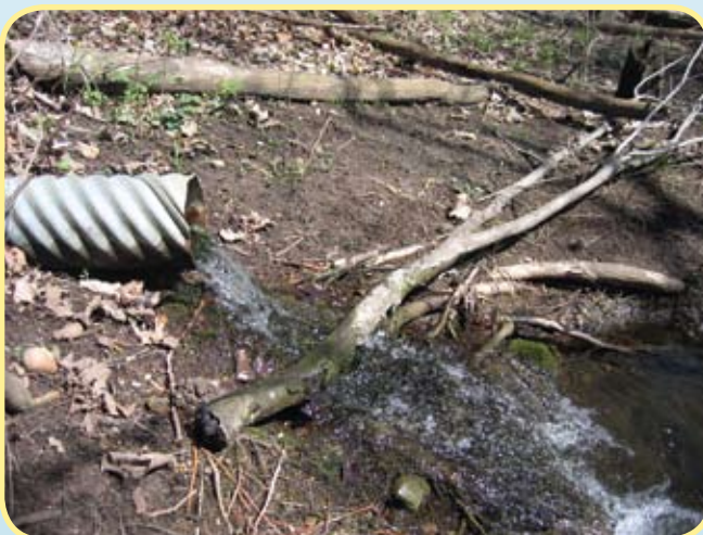
Figure 7 - Stormwater runoff entering a stream
