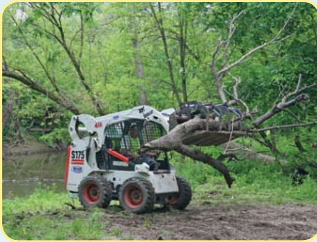
Figure 11 - If conditions allow, a small skid steer or tractor may be used to remove LWD
