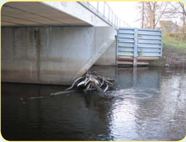
Figure 40 - Minor LWD accumulation on bridge pier
