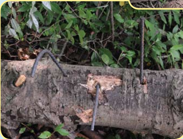
Figure 33 - Bend rebar to secure log in place. The easiest way to bend rebar is to apply leverage to the top of the bar after it has been pounded into the woody debris and substrate.
